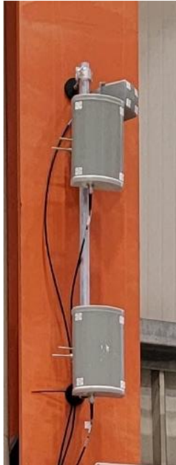
Figure 4-2: LocataLite with Indoor Wall (180° Coverage) Antennas
